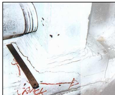
Crack highlighted by dye penetrant inspection
